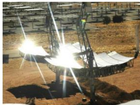
Dish Collectors at Sandia
